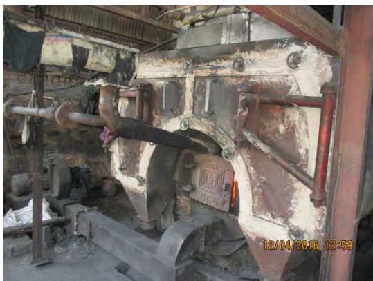
Caption: Steam boiler at Simandhar Fabtex
