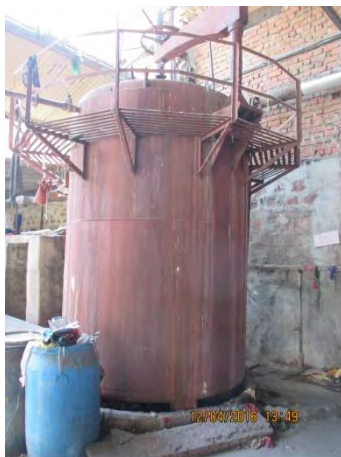
Caption: Kier Boiling unit at Simandhar Fabtex
